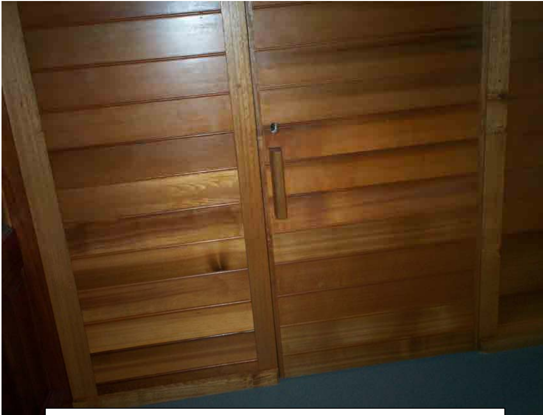
This door leads into a staff area near a lounge. The doors are disguised the same as the walls with only the keyhole and handle showing it is a door.
